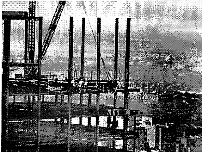
Ironworkers, such as those pictured here on the construction site of Philadelphia's Fidelity Mutual Life Building in 1970, belonged to one of the city's most racially exclusive unions. In the summer of 1969, the U.S. Department of Labor found that only 1.4 percent of ironworkers in the Philadelphia area were nonwhite. Courtesy Temple University Libraries, Urban Archives, McDowell Bulletin Collection.
